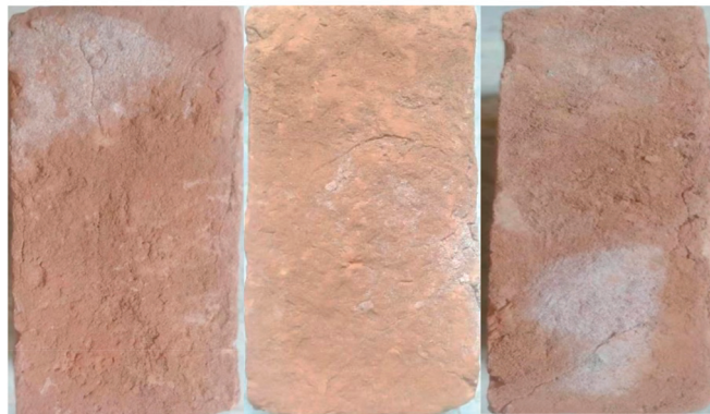
Figure 8. The effect of efflorescence.
