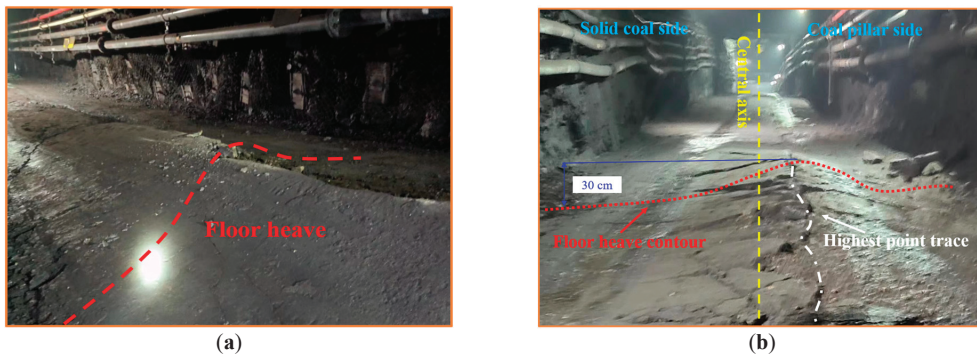
Figure 2. Failure characteristics of the roadway floor. (a) Floor heave; (b) Asymmetric floor deformation.
