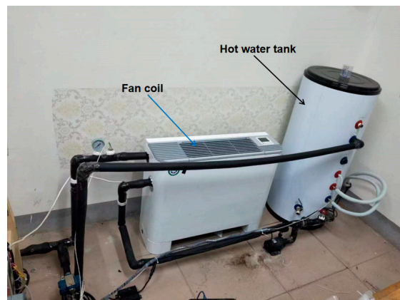
Figure 3. Fan coil and hot water tank.
