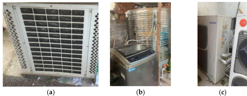
Figure 3. Photos of home hotel energy-using equipment: (a) air source heat pump as a water heater; (b) electric water heater; (c) air source heat pump for air conditioning.
