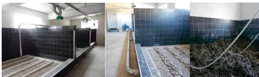
Figure 1. Aerated static pile composting system.
