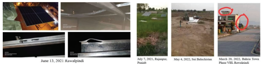
Figure 1. Damages caused by wind to solar PV mounting structures at different locations. Red mark shows the damaged solar PV mounting structure.
