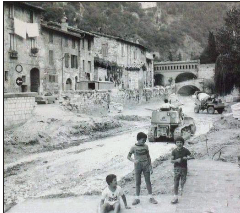
Figure 22. The paving works of the riverbed of the Camignano Creek (around the end of 1970s) in a photo from the time.
