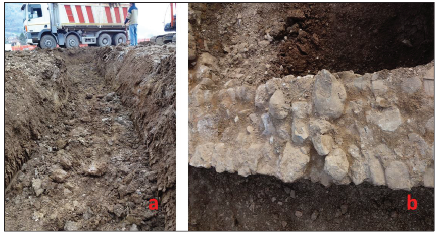
Figure 8. (a) The trench made during the excavation of the building in Figure 7; (b) pebbles of clear fluvial origin used to build the artifact.
