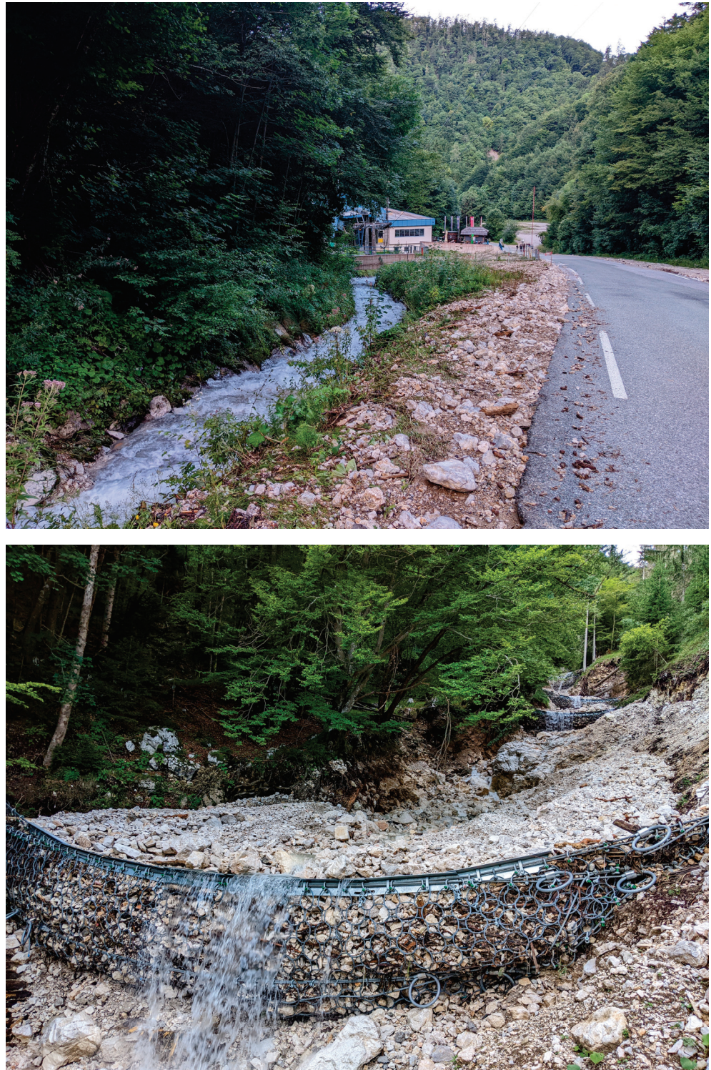
Figure 13. A situation in both torrents after the extreme August 2023 event.
