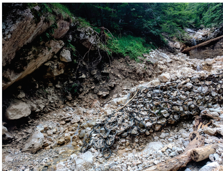
Figure 5. One example of the consequences of the May 2018 event on the existing infrastructure in both torrents: a partially destroyed already filled flexible barrier.
