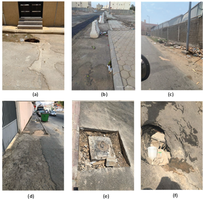
Figure 1. Examples of the three categories central to this study: (a,b) represent the barrier category, (c,d) illustrate the sidewalk category, and (e,f) depict the pothole category. All RGB images were collected from Saudi Arabia.
