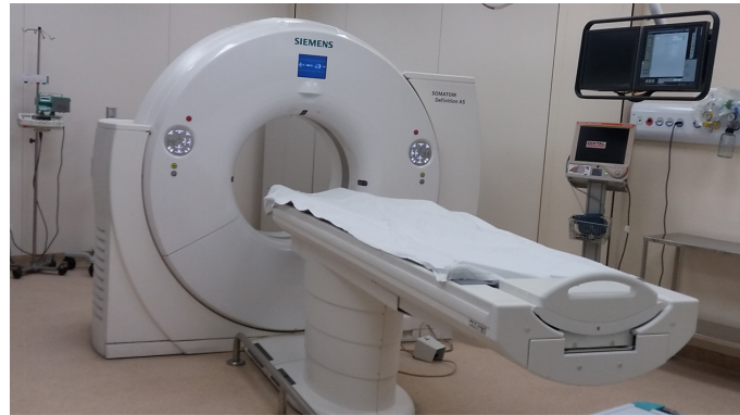
Figure 17. MRI/CT scanner room.
