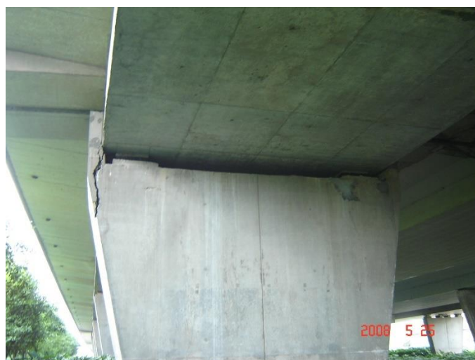
Figure 3. Anti-knock block failure because of transverse deformation of the girders.
