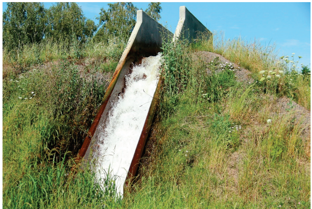
Figure 2. Cascade (staircase) behind the inflow of mine water to the treatment plant.
