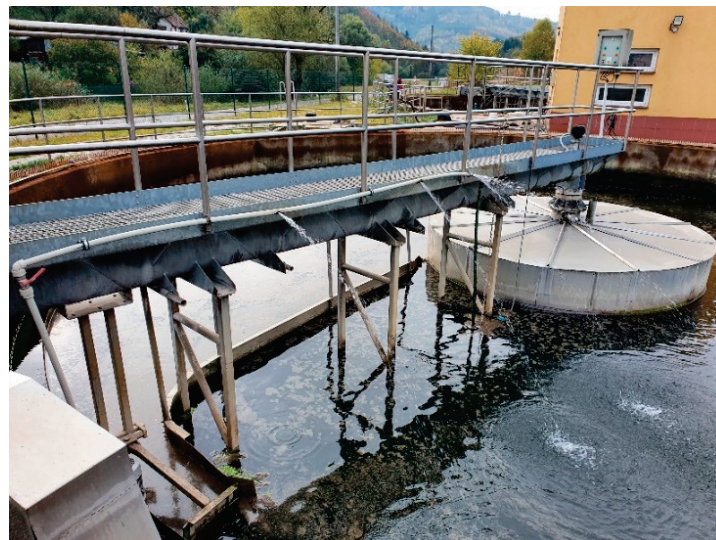
Figure 1. Spread of floating sludge.
