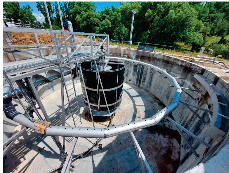
Figure 2. New mechanical and technological equipment of the settling tank.
