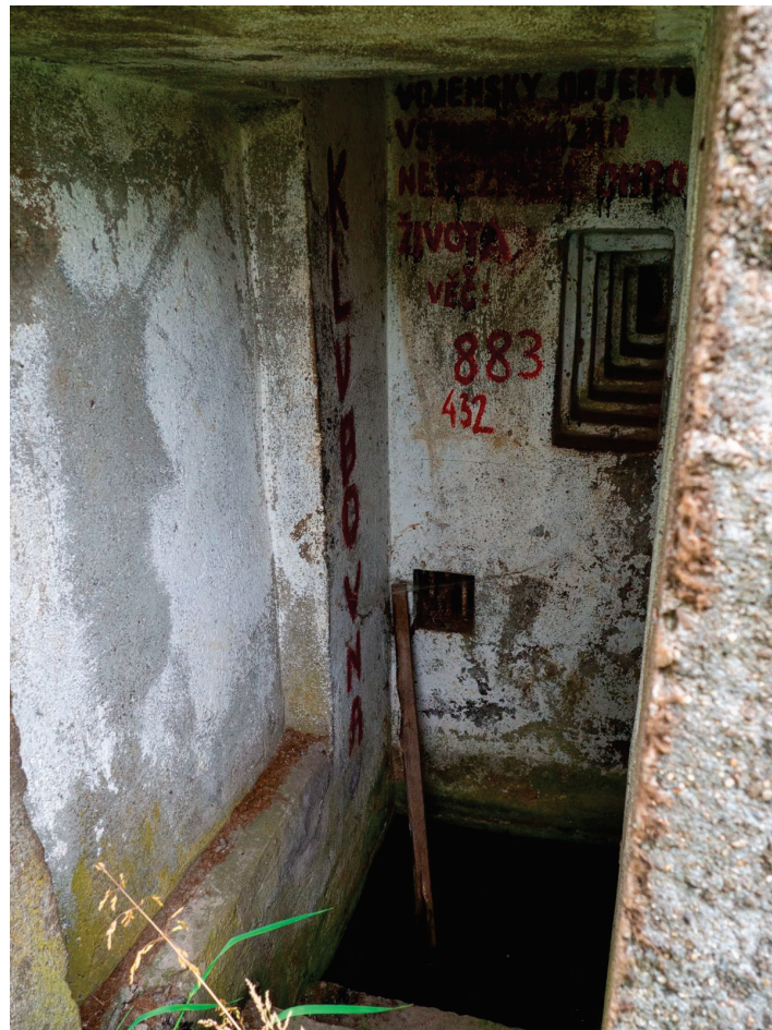
Figure A2. Inscriptions “Klubovna” (“Clubhouse”) next to the warning sign “Vstup zakázán, nebezpečí ohrožení života” (“Entry forbidden, danger to life”) can be seen like UMF-C’s “hidden curriculum”. Author: Adéla Brázdová.
