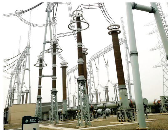
Figure 3. The 1000 kV surge arrester with supporting structure installed in an UHV electrical substation.
