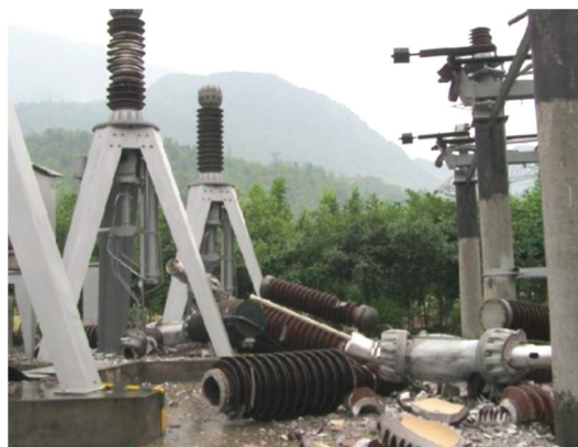
Figure 1. Seismic failure of porcelain insulators in the M7.9 Wenchuan earthquake in 2008.
