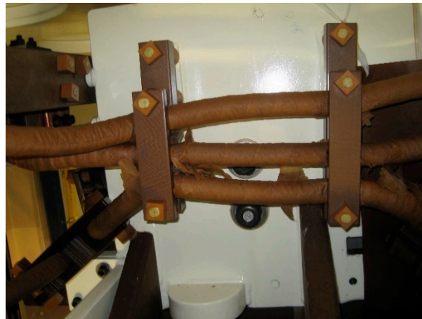
Figure 1. Damaged insulation during short circuit test.
