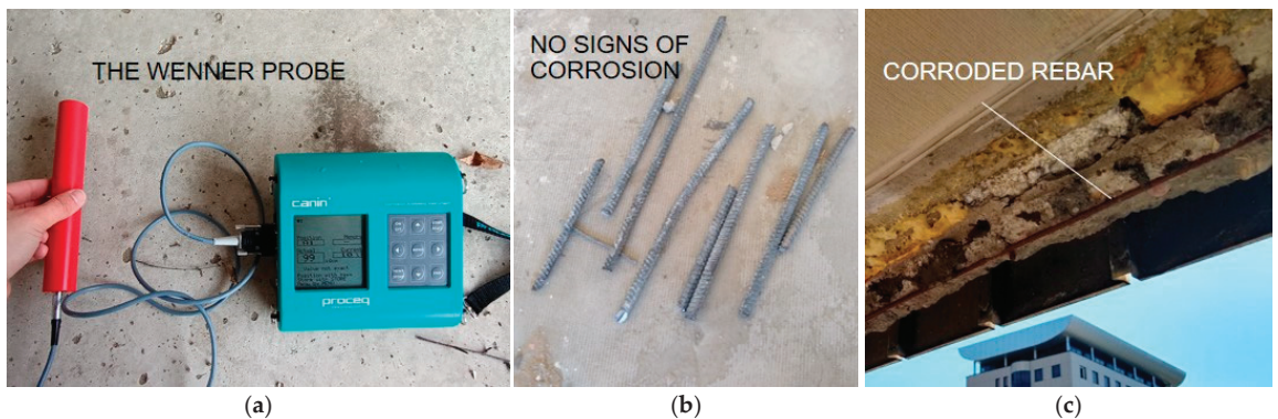
Figure 11. Corrosion investigation of reinforcing steel: (a) Wenner probe test; (b) visual inspection of rebars from excavations; (c) exposed corroded beam-wall rebar.
