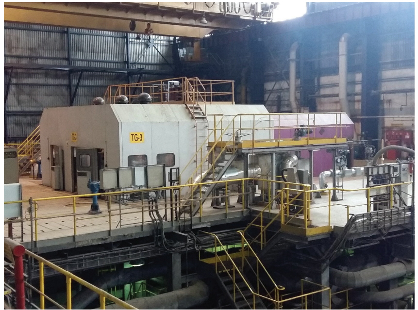
Figure 1. General view of a turbogenerator.
