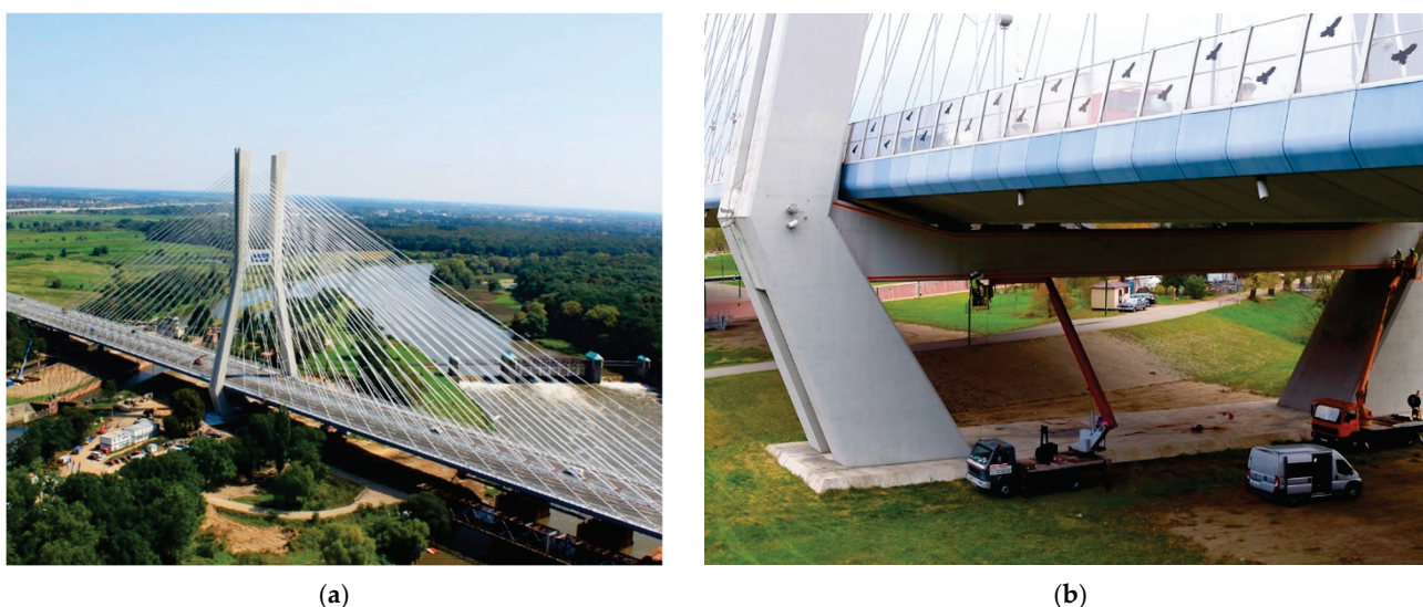
Figure 19. (a) Rędziński Bridge in Wrocław, Poland—general view (photo: W. Kluczewski); (b) the close-up of the lower crossbeam connecting two inclined legs of the pylon.
