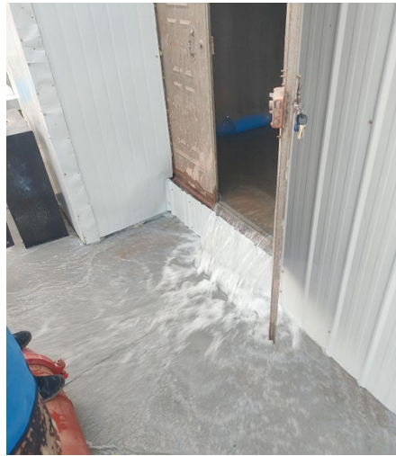
Figure 17. Ruptured pipe on site.
