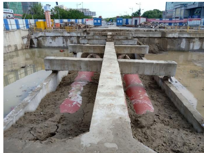
Figure 2. A photograph of the pipelines in the YRNE Project.
