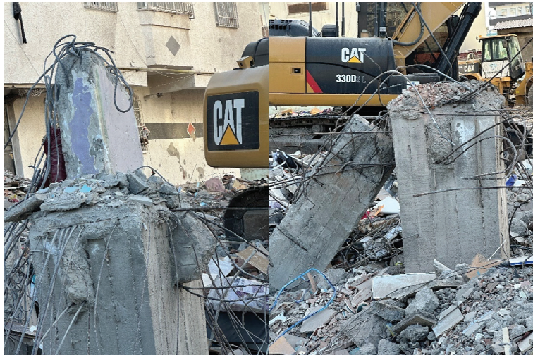
Figure 8. Retrofitting of the ground floor only and the failure of the old column.
