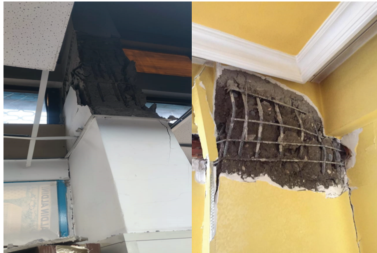
Figure 10. Damage to the short column and shear wall with poor concrete.
