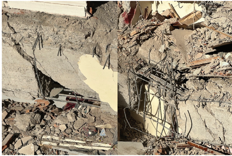
Figure 7. Shear damage of the beam and inappropriate stirrups.
