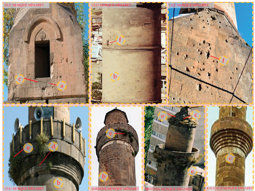
Figure 4. Damages observed in Five Minarets: a. high temperature difference; b. discoloration and color change; c. water effects; d. rupture damage; e. vegetation and f. bullet traces.
