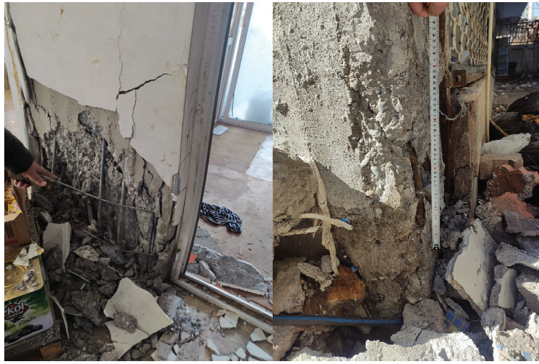
Figure 9. Extensively damaged columns.
