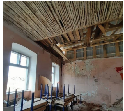
Partial collapse of the floor structure
