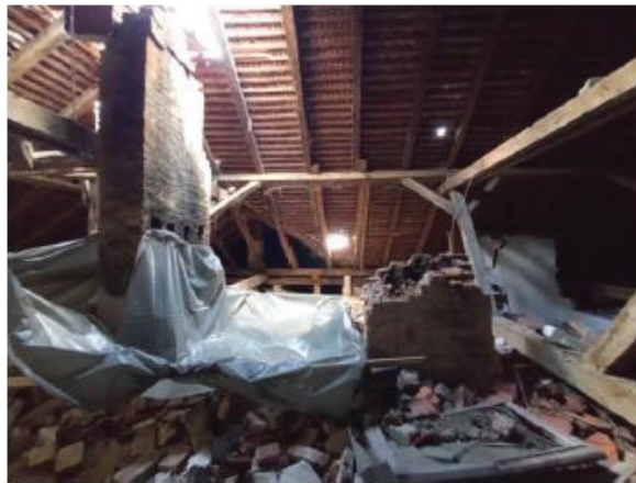
Figure 11. Collapsed chimney and damaged roof covering.
