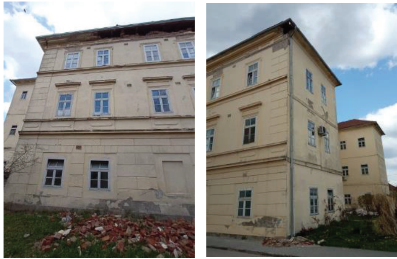
Figure 10. Damage to the facade.
