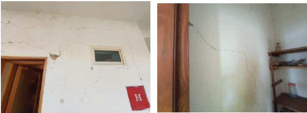
Figure 8. Cracks on the load-bearing walls on the first floor.
