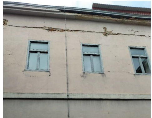
In-plane sliding failure (horizontal cracks)
