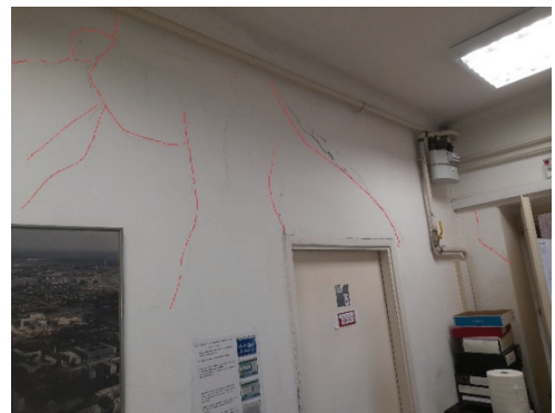
(b) First floor damage
