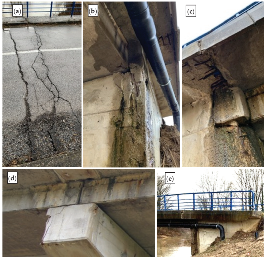
Figure 14. Hader bridge: (a) damage caused by earthquake in the asphalt; (b) fractured abutment side wall due to the earthquake; (c) water leakage from superstructure end, causing damage to abutment; (d) uneven support length for the girders; (e) cracked cornice due to earthquake movement.
