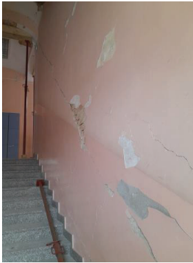
In-plane shear failure of interior walls
