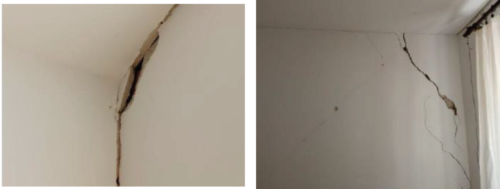
Figure 9. Cracks at the junctions of load-bearing walls.
