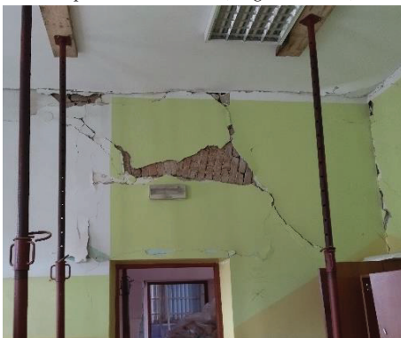
Shear failure of spandrels (diagonal cracks)
