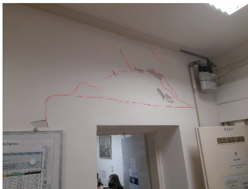
(a) Ground floor damage
