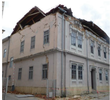
Partial overturning of the gable walls
