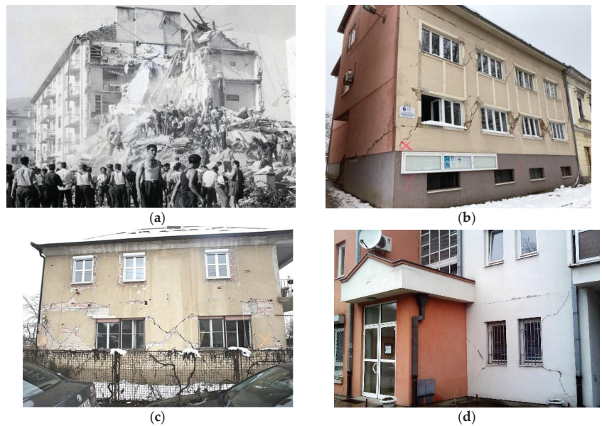
Figure 2. Seismic performance (DSs) of URM residential buildings in past earthquakes in the Balkan region: (a) DS5—a collapsed building in Skopje due to the 1963 Skopje earthquake (credit: Z. Milutinović); (b) DS4—a URM building in Petrinja experienced extensive cracking in wall piers due to the 2020 Petrinja earthquake (credit: SUZI-SAEE); (c) DS3—a URM building in Petrinja experienced a major shear-induced cracking in piers at the ground floor level due to the 2020 Petrinja earthquake (credit: SUZI-SAEE), and (d) DS2—a moderately damaged URM building which experienced moderate shear-induced cracking due to the 2010 Kraljevo earthquake (credit: P. Blagojević).
