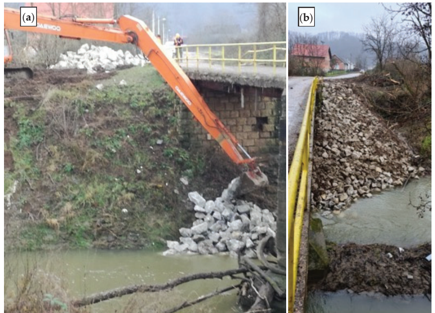
Figure 15. Immediate measures to secure the abutment of Matija Gubec street bridge: (a) beginning of the work; (b) completed infill.
