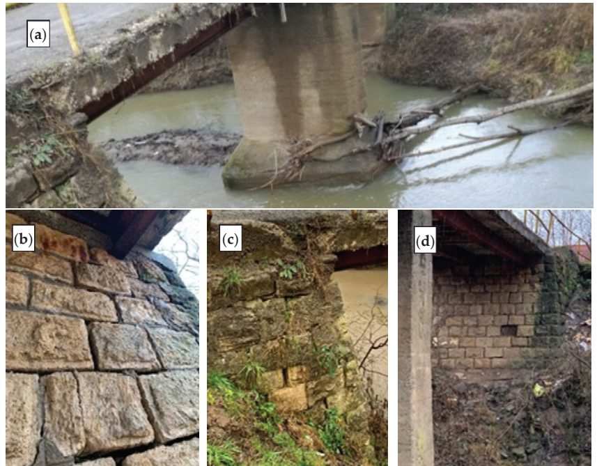
Figure 8. Matija Gubec street bridge: (a) columns—large foundation for the column in the middle of the riverbed and scour visible on the east column; (b) abutment stone wall damage; (c) abutment sliding signs; (d) evidence of subsequent abutment sliding—stone wall integrity compromised.
