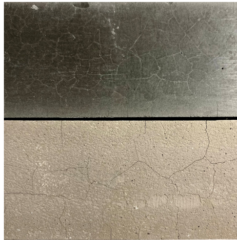
Figure 6. Cracks of specimens caused by plastic shrinkage (above) and drying shrinkage (below).
