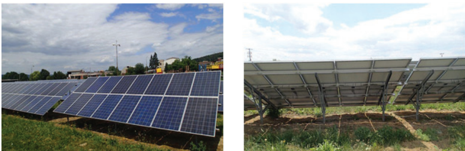
Figure 2. Experimental PV power plant with PV modules PHONOSOLAR PS240P–20/U.
