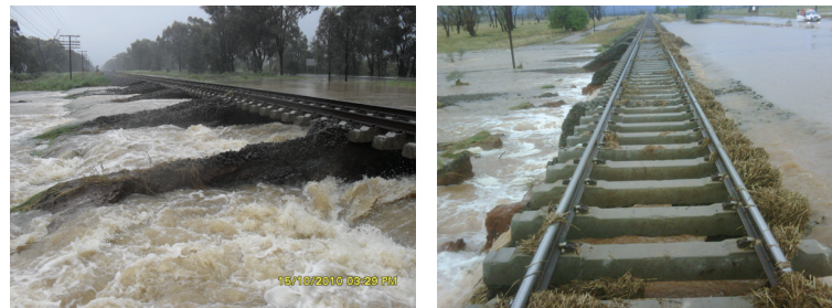
Figure 1. Scouring of railway ballast during flooding in the Hunter Valley, NSW, Australia, in October 2010. Copyright Australian Rail Track Corporation.
