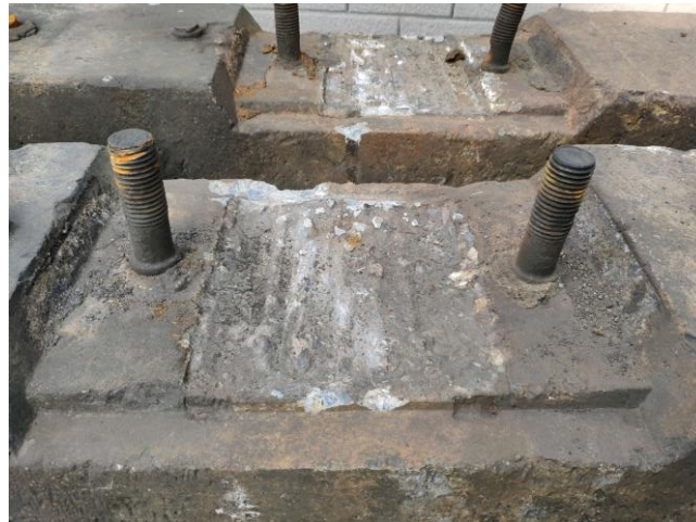
Figure 18. Concrete sleeper rail seat abrasion.
