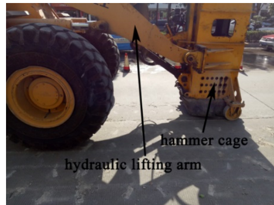
Figure 1. Micro-crack homogenization crushing of pavement structure [2].
