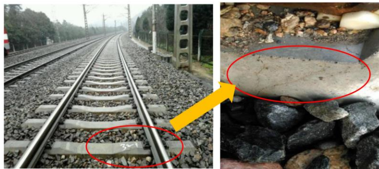
Figure 19. Transverse crack in the rail seat section of the concrete sleeper.
