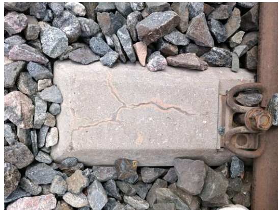
Figure 11. AAR damaged the concrete sleeper. Note: These images also show other factors in addition to AAR.
