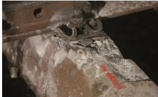
Figure 13. Damaged concrete sleeper in the derailment.
