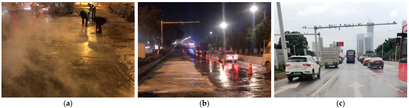
Figure 2. Applications of rapid-hardening HSFRC in practices. (a) Casting of concrete. (b) Hardening of concrete. (c) Operation situation for 3 years.
