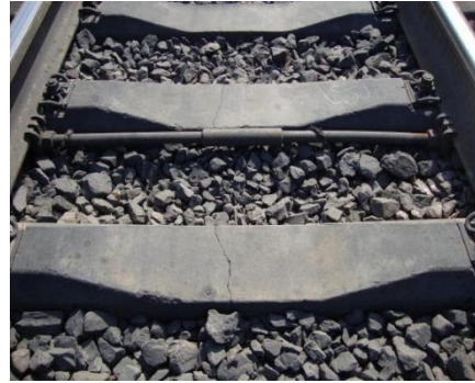
Figure 16. Track bed hardening damages the concrete sleeper.
