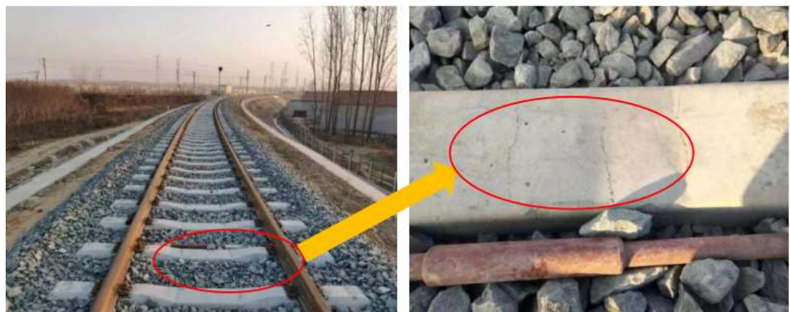
Figure 20. Transverse crack in the central section of the concrete sleeper.
