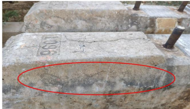
Figure 21. Horizontal crack on the side of the concrete sleeper.
