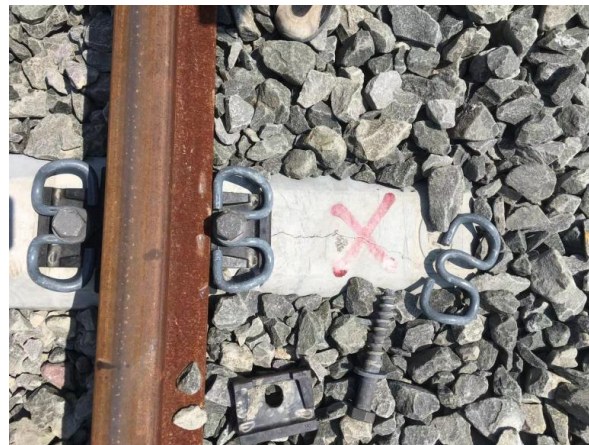
Figure 14. Excessive torque of the buckling bolt causes sleeper damage. Note: These images also show other factors in addition to the torque of the buckling bolt.
