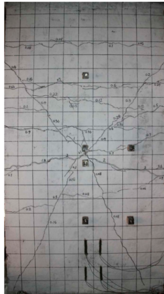
Figure 12. Cracks at the back of the RC shear wall [14]. Copyright 2019, Vibration and Shock.
