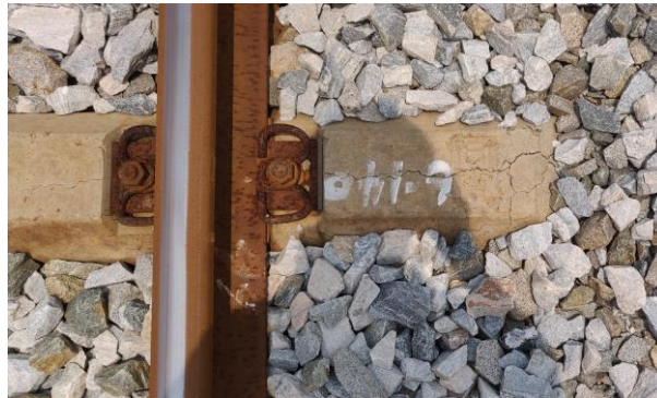
Figure 12. DEF damaged the concrete sleeper. Note: These images also show other factors in addition to DEF.
