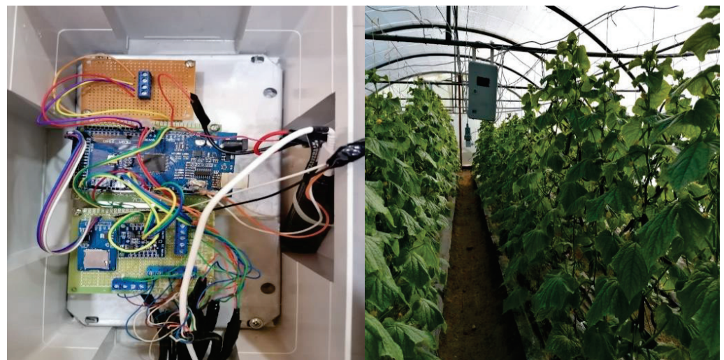
Figure 2. Actual prototype of the Arduino microcontroller system installed inside the greenhouse.
