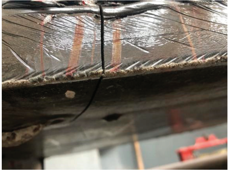
Figure 9. Fracture of L1 polyurethane.
