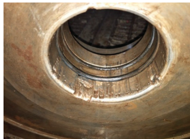
Figure 3. Eccentric wear phenomenon on the inner wall of the main diameter of a BOP.
