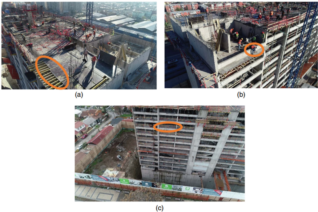
Figure 6. UAV images for safety monitoring at a construction site in Chile: (a) lack of guardrails; (b) worker without safety rope; and (c) lack of guardrails (Images by Jhonattan G. Martinez) [92].
