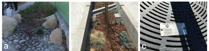
Figure 4. Examples of Los Angeles systems designed to remove debris and contaminants from runoff: (a) biofilter along Elmer Avenue Paseo, (b) biofilter in the Avalon Green Alley, and (c) Filterra™ bioretention system on Grand Boulevard.
