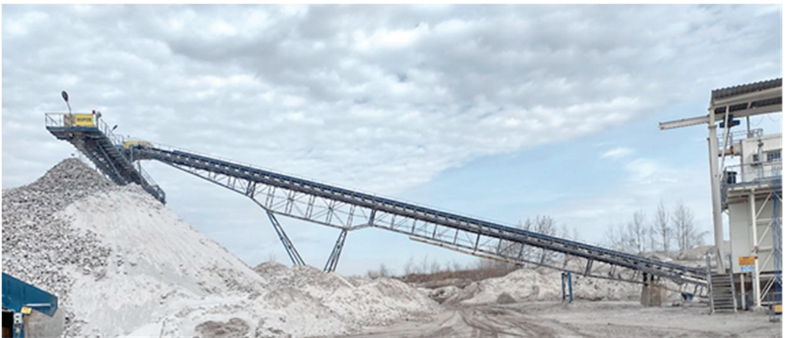
Figure 1. Belt feeder in the technological line of the processing plant of an aggregate mine.
