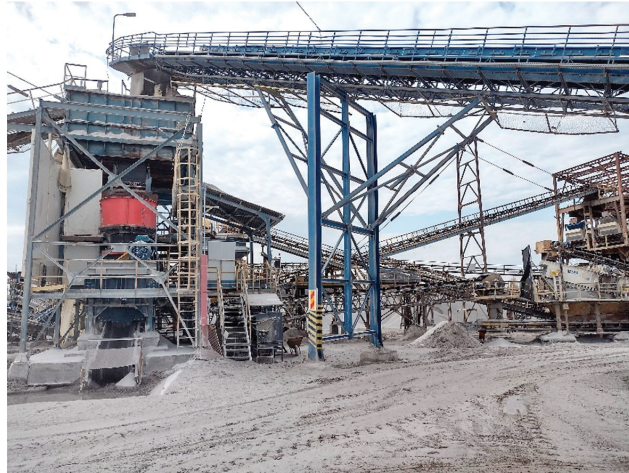
Figure 8. Belt feeder with SSSs (straight stationary supports).
