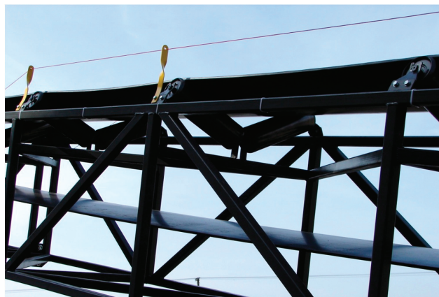
Figure 4. Belt feeder's route with idlers, trestles, and a safety line.
