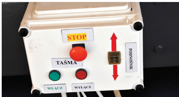
Figure 7. Local control of the belt feeder.
