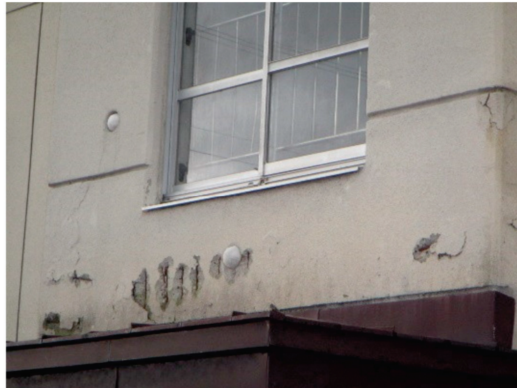
Figure 3. Spalling of concrete due to cracking and corrosion in a cold climate [107].
