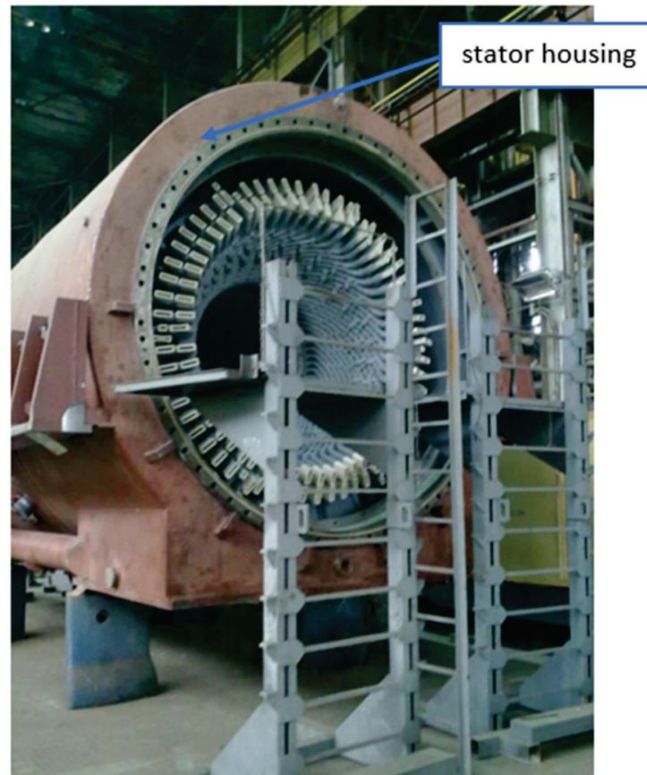
Figure 6. The Stator of Turbogenerator TGV-300-2U3.
