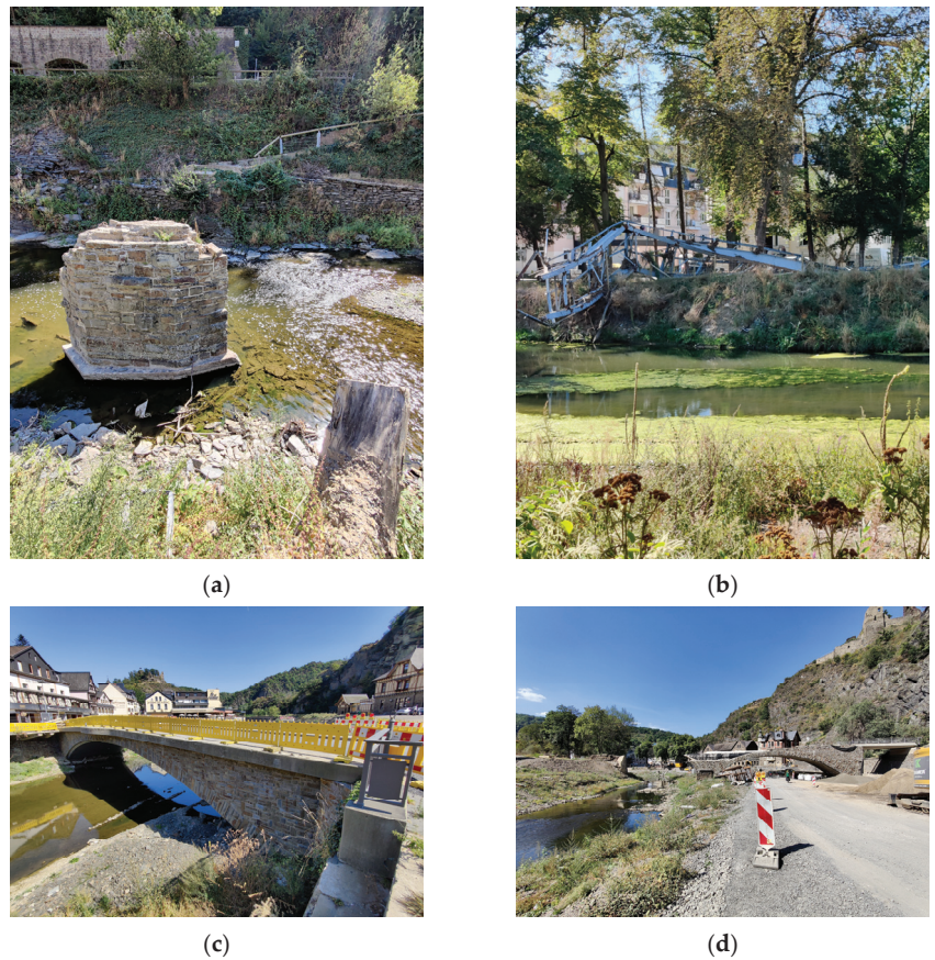
Figure 6. Surveyed overtopping mechanisms: (a) remaining pier of a dragged wooden deck; (b) girder of a dragged steel deck; (c) damaged railing due to overtopping; (d) combination of overtopping and scour, with the latter being responsible for triggering the failure. Pictures taken by the first author.
