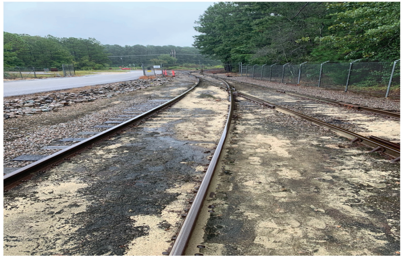
Figure 1. Fouled Ballast located at an Army Installation.
