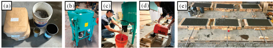
Figure 1. Construction of TARUHPC specimen: (a) batching, (b) high-shear mixture, (c) discharging UHPC, (d) pouring UHPC, (e) after pour.
