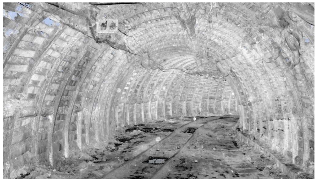
Figure 3. Point cloud view of the mine tunnel straight section near the bend.
