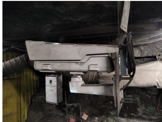
Figure 2. Measuring equipment—RGB camera to monitor the working conditions of the transfer point.
