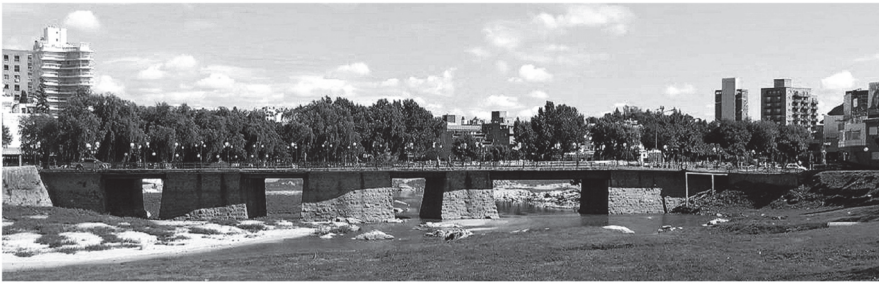
Figure 2. The existing 1889 bridge, its supporting piles account for 45% of the drainage section. (Credit: Reproduced with permission from the author, Eng. Gerónimo Cáffaro).
