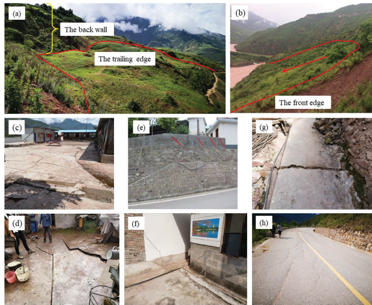
Figure 10. Field survey photos. (a) The trailing edge has sunk. (b) The front edge has slid. (c) Cracks in the Cheyiping primary school. (d) Cracks in villagers’ homes. (e) Fissures in the walls. (f) Cracks in houses. (g) Cracks in the road in the village. (h) Deformation of Bao–Tibet highway.
