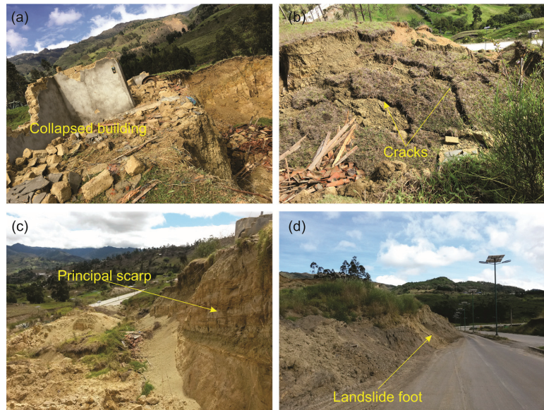
Figure 2. (a) Collapse of houses due to slope movement activity; (b) Presence of cracks in the slope body; (c) View of the main scarp on the southern flank of the slope; (d) Accumulation zone along the roadway.
