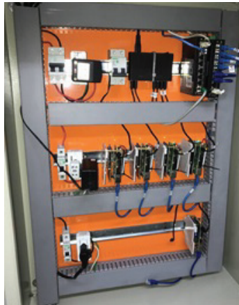
Figure 15. Supervisory system hardware box.
