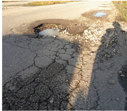
Figure 1. Pavement deterioration, with alligator cracking, after very heavy rainfalls during the winter (Portugal).
