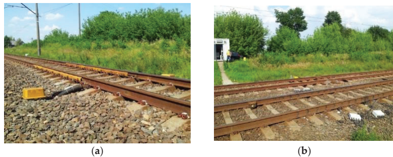
Figure 6. Used measurement systems: (a) regular system ATLAS-LG; (b) specially designed system IC VEIP.
