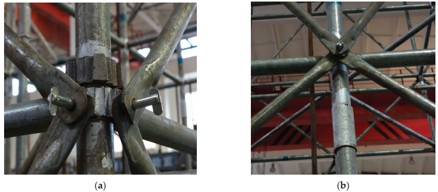
Figure 3. Detail of rod-end connection. (a) Connection of upright rods with horizontal rods and diagonal rods. (b) Connection of upright rods.
