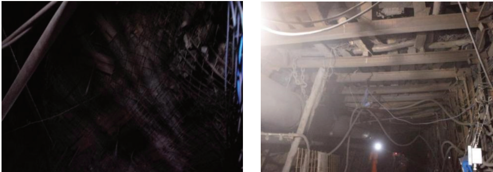
Figure 4. Deformation of surrounding rock during roadway excavation.
