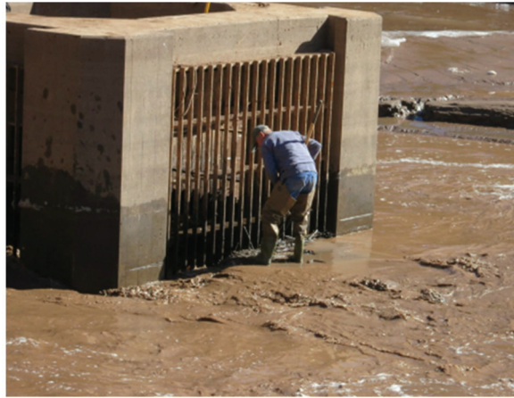
Figure 6. Paonia Dam water diversion outlet structure partially blocked by sediment (USBR photo taken on 11 November 2014).
