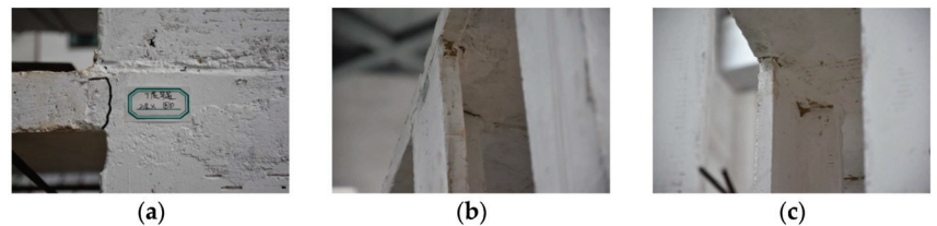
Figure 9. Damages after excitations of the rare level of intensity 7 (Phase III): (a) an extended interface crack; (b) slight crushing of a T-shaped wall; (c) interior view of the structure.
