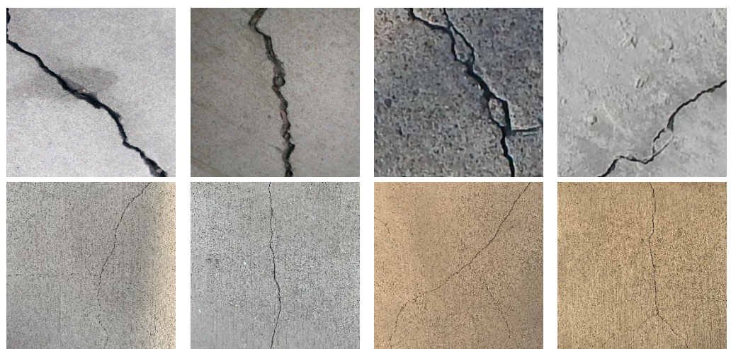
Figure 1. Comparison of crack features. The first row shows images of cracks in the open dataset [31,39], and the second row shows images of cracks in concrete dam surfaces.
