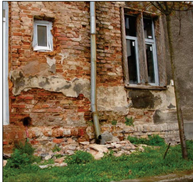
Figure 3. Damage to a plaster and brick wall due to leaking drainpipes.
