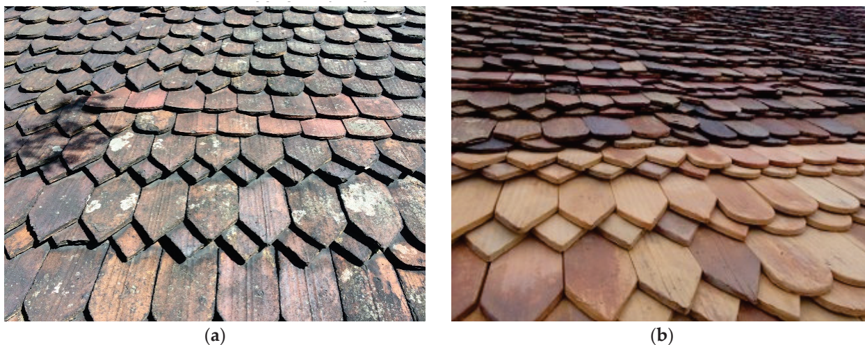
Figure 14. Different types of roof tiles: (a) historical; (b) new roof tiles in historic dimensions.
