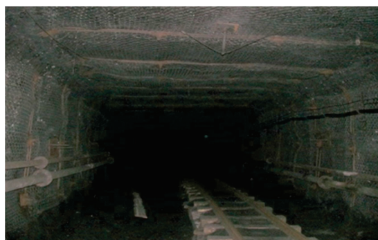
Figure 17. Real picture of deformation control effect of reserved roadway surrounding rock.
