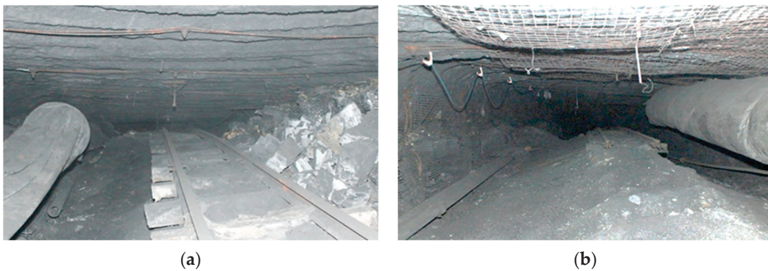
Figure 2. Real pictures of surrounding rock deformation of 1523103 roadway. (a) Roof subsidence; (b) bottom drum situation.
