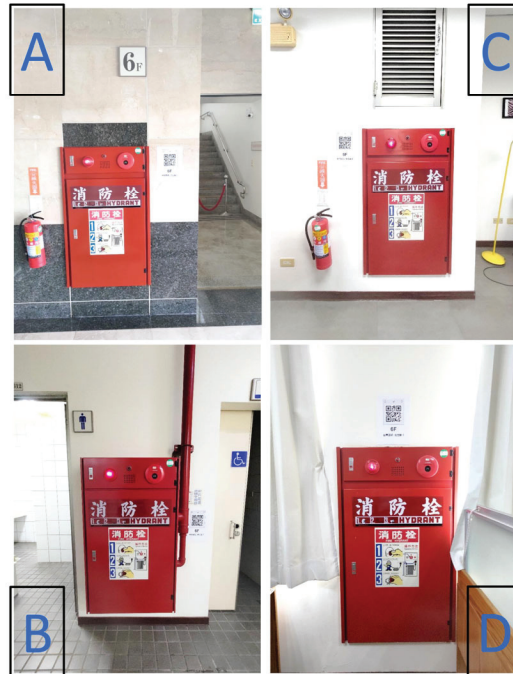
Figure 4. The photos of the four fire hose hydrant boxes labeled with A, B, C, and D in Figure 3.
