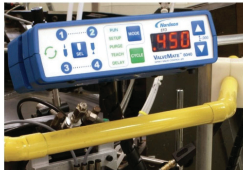
Figure A2. Controller operation panel.
