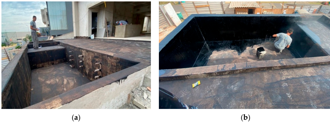
Figure 7. (a) Pool with primer applied; and (b) use of modified asphalt on the pool surface.
