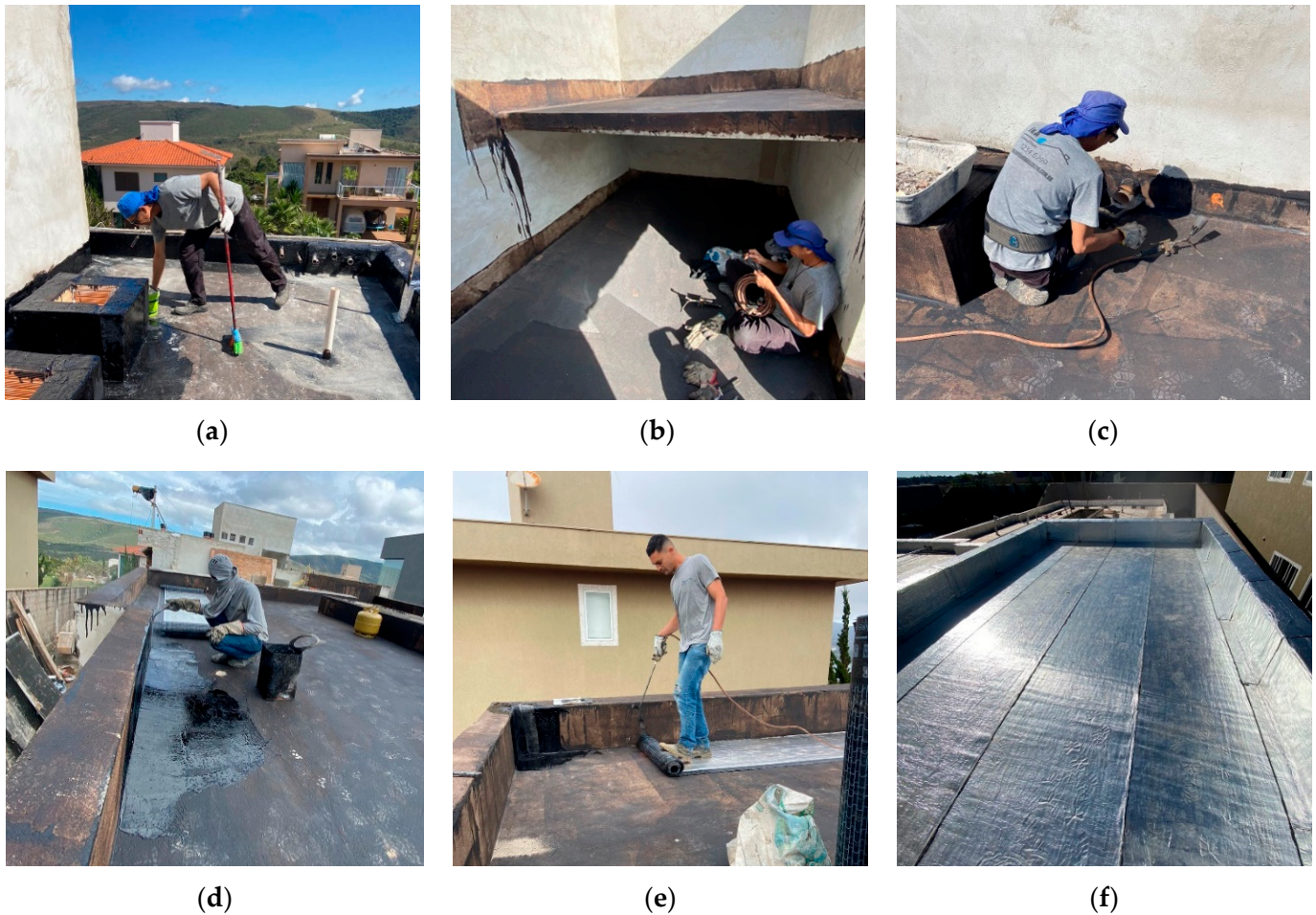
Figure 5. (a) Primer application on the slab; (b) primer application in water tank room; (c) use of a blowtorch to melt the modified asphalt; (d) application of modified asphalt to receive the blanket; (e) positioning of the blanket roll on the slab; and (f) aluminized asphalt blanket applied on the slab.
