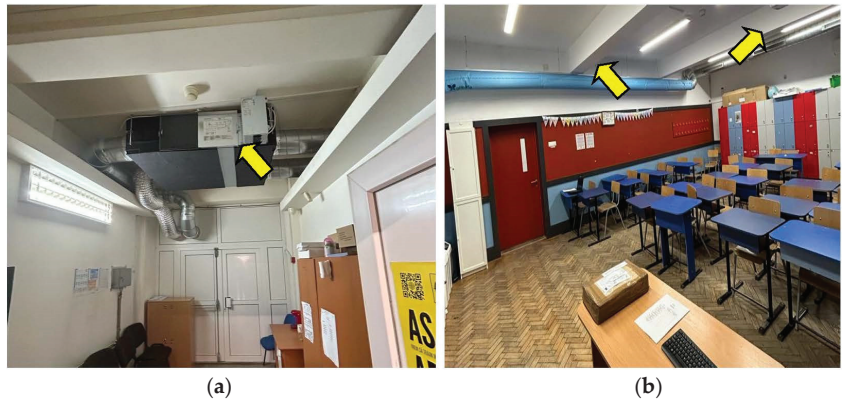
Figure 2. (a) Heat-recovery unit placed in the school hallway. (b) Textile introduction of fresh and extraction with regular HVAC duct.
