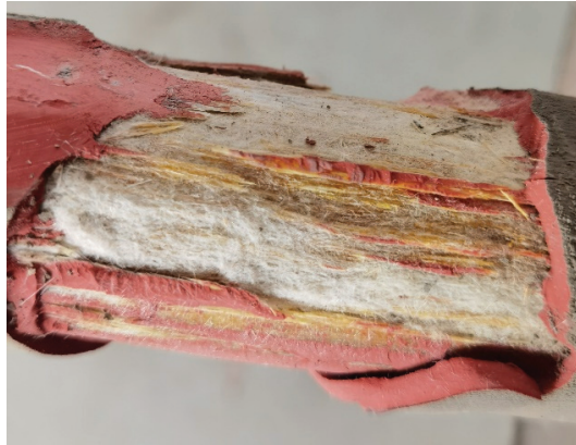
Figure 5. Debris at the core rod–sheath interface of a brittle composite insulator.
