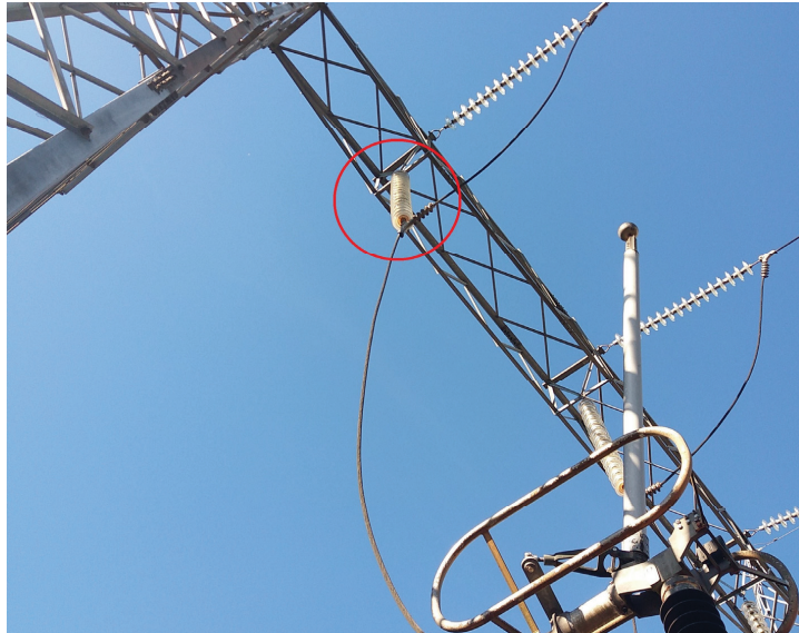
Figure 22. In this insulation chain of 230 kV, superficial-type partial discharge was found to be present specifically in phase A.
