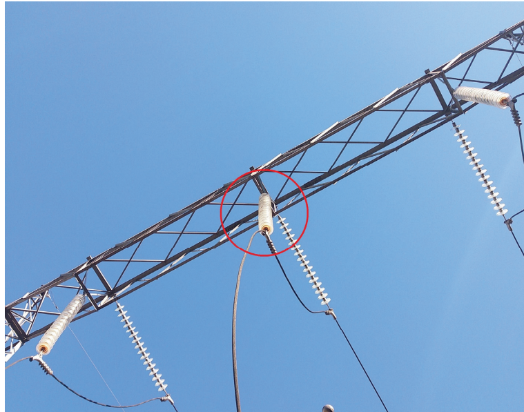
Figure 21. In this insulation chain of 230 kV, corona-type partial discharge was found to be present specifically in phase B.
