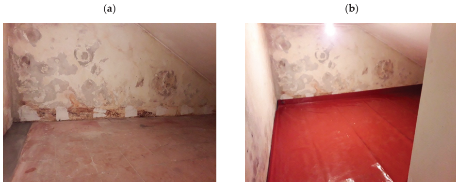
Figure 6. Placement of the Rn barrier membrane. (a) Floor before placing the barrier membrane; (b) Floor after placing the barrier membrane.
