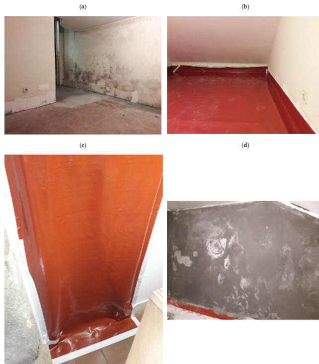
Figure 4. A sequence of works carried out. (a) Initial appearance before the execution of the tasks; (b) barrier membrane application; (c) sealing of the outer compartment door; (d) application of mortar to the compartment walls.
